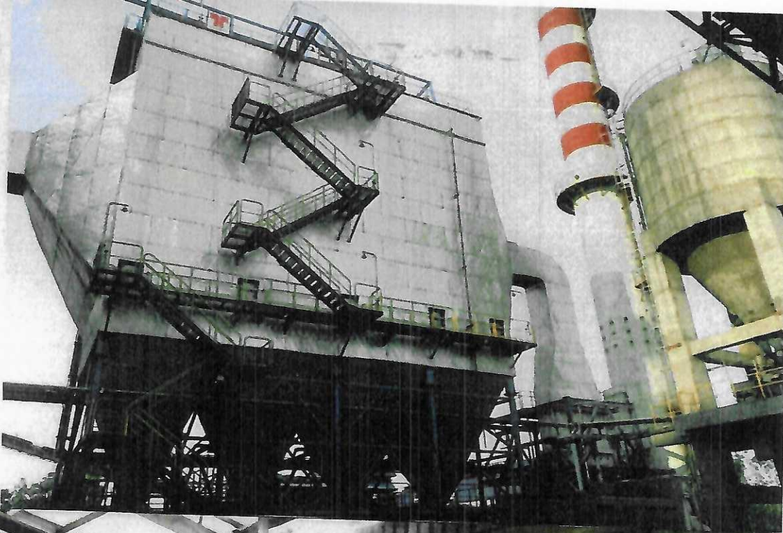
Photograph showing installation of ESP connect to the stack of Power Plant.
